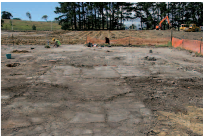
2. The upper terrace building platform with the lower terrace concrete pad in the foreground.
