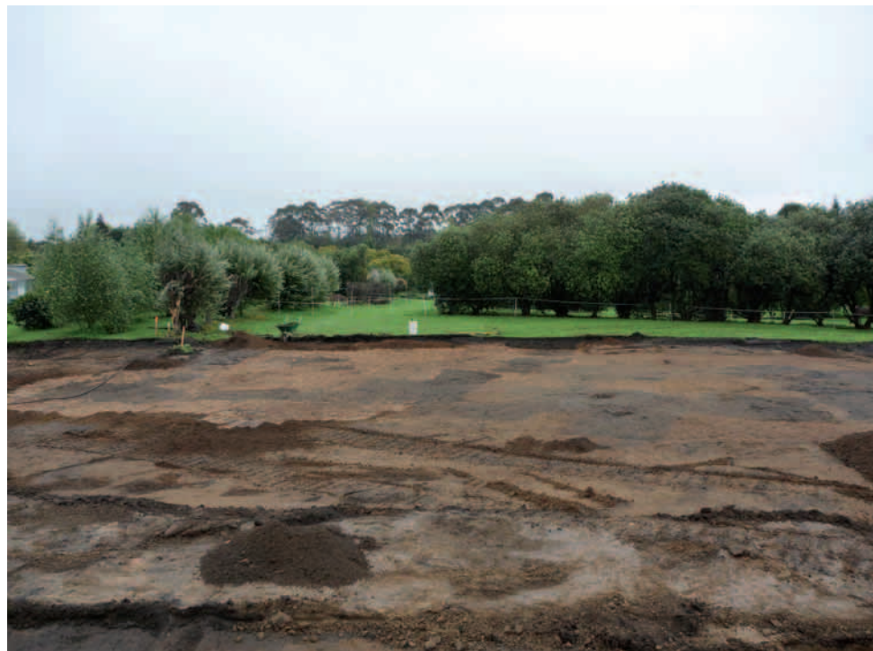
2. General view to the northwest after the topsoil has been removed. The pits are visible as dark rectangles against the lighter coloured subsoil.
